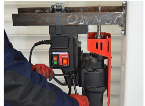
Out of position drilling
